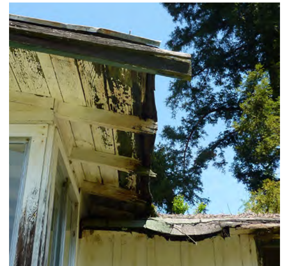
Figure 323. Deteriorated sheathing and rafters.
