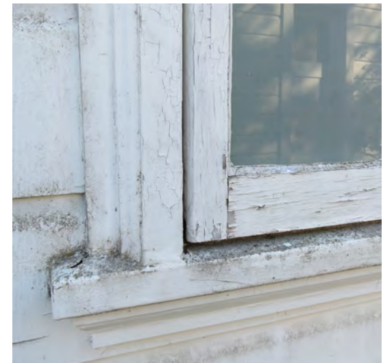
Figure 170. Wood window with paint loss and glazing compound deterioration.
