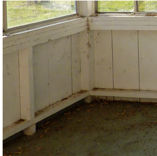
Figure 339. Enclosed Porch with worn carpet.
