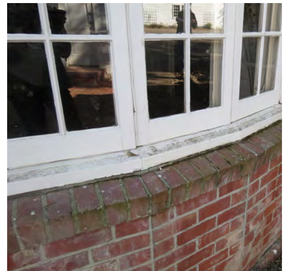
Figure 90. Biological growth on bricks and window sill.
