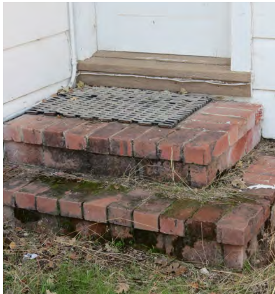
Figure 229. Brick steps with heavy biological growth and deteriorating mortar.
