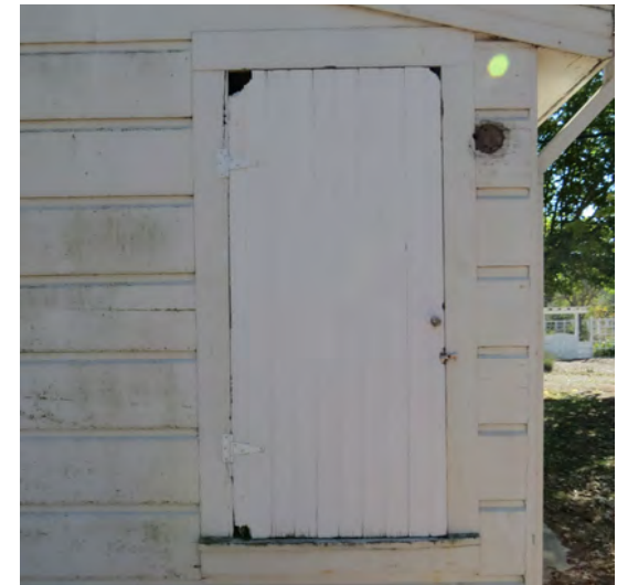
Figure 284. Wood deterioration at half size door.
