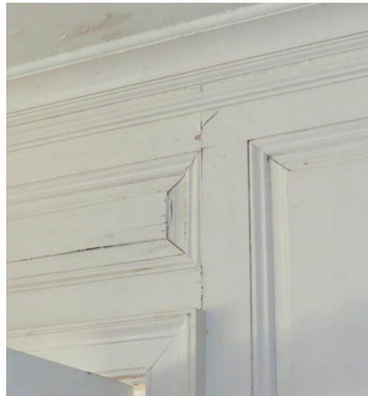
Figure 97. Water damaged painted wood paneling in Room 104.
