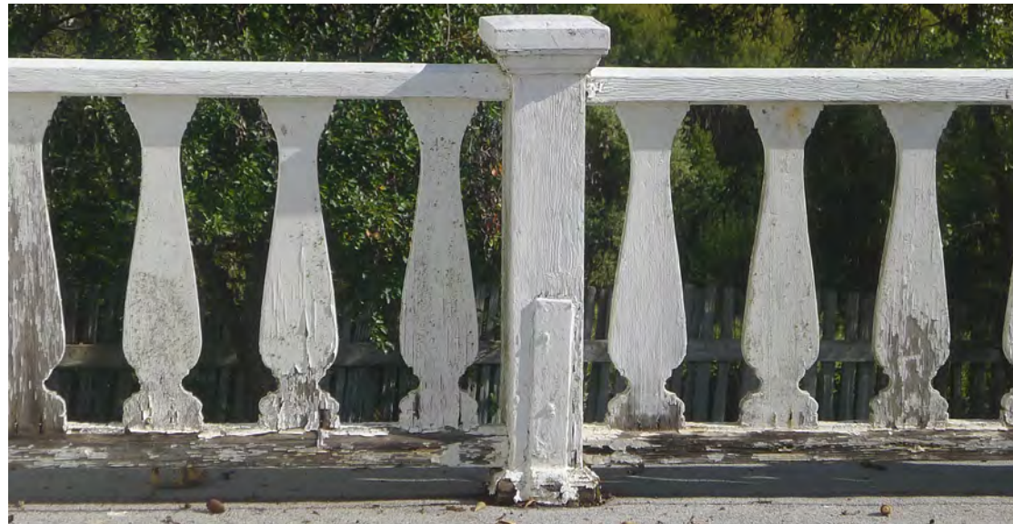
Figure 84. Severely damaged wood railing at balcony.
