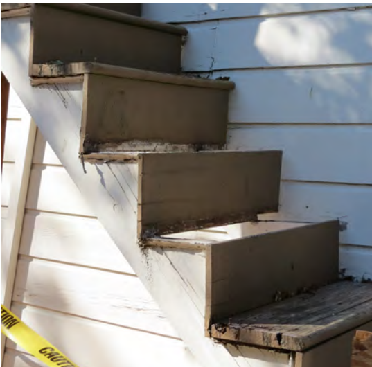
Figure 137. Deteriorating wood stair.
