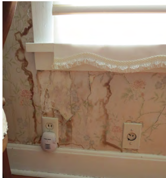
Figure 100. Water damage below window in Room 109.
