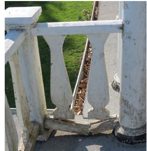
Figure 86. Broken piece of balcony railing.
