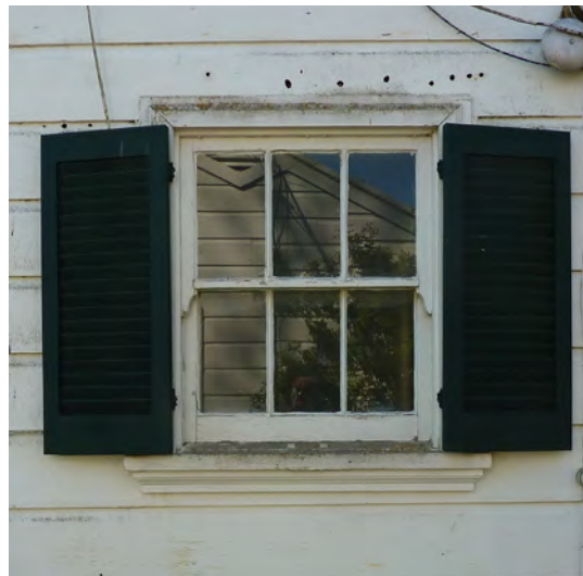
Figure 169. Double hung window with biological growth covering trim and shutters in good condition.
