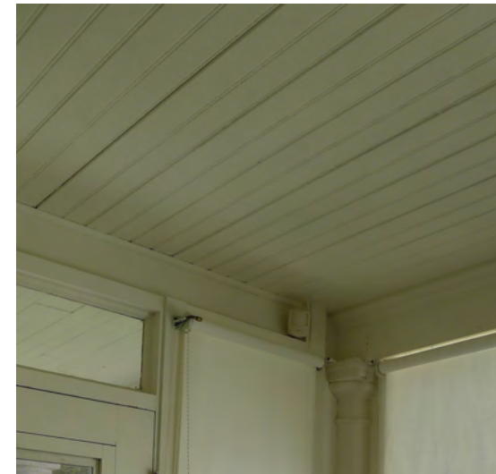
Figure 104. Painted bead board ceiling in Room 108, a portion of the original porch.
