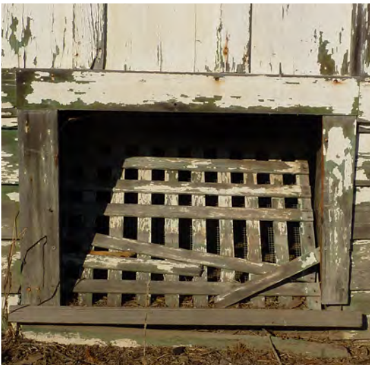
Figure 337. Damage vent at foundation where pests can enter the crawl space area.
