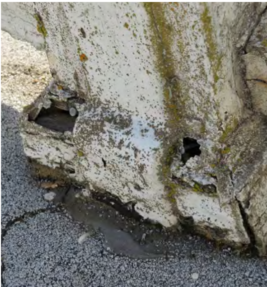
Figure 83. Deteriorating base of railing post.
