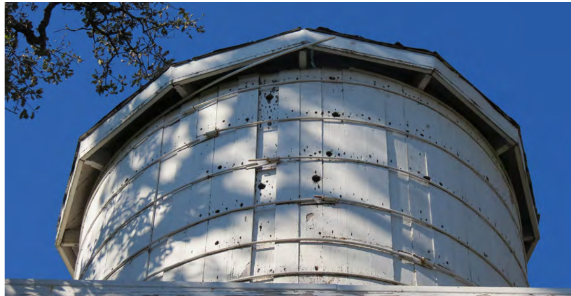
Figure 130. Woodpecker holes at tank boards.
