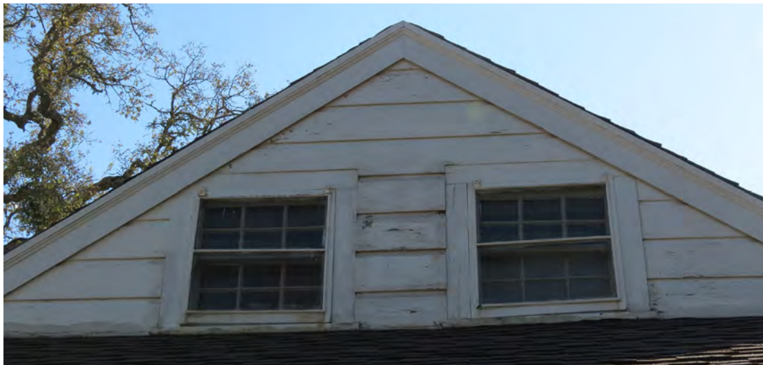
Figure 286. Windows with trim deterioration.
