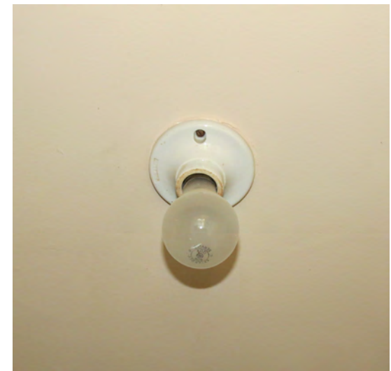
Figure 118. Common ceiling mounted light fixture.
