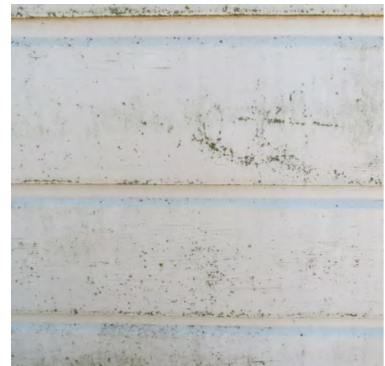
Figure 293. Biological growth on painted siding.
