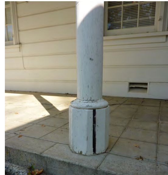
Figure 228. Wood column with damaged base.
