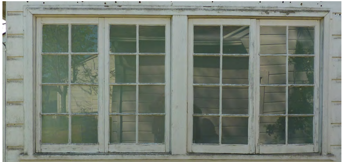
Figure 168. Wood casement windows with paint loss and biological growth.
