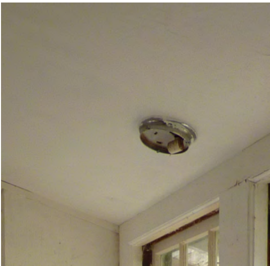
Figure 353. Light fixture in Kitchen.
