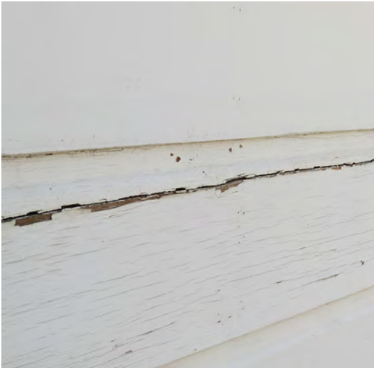
Figure 72. Longitudinal split in siding.
