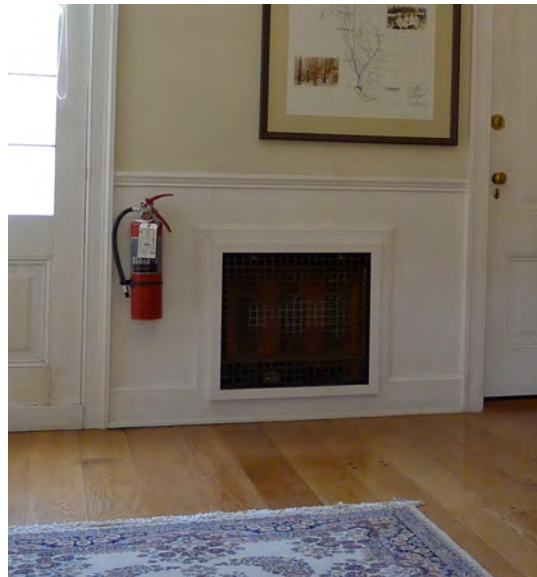
Figure 123. Wall mounted electric heater in Stairhall 201.
