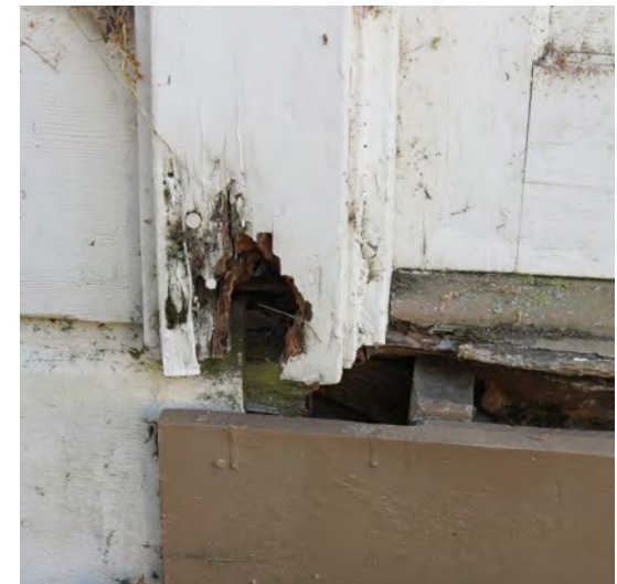
Figure 226. Deteriorated wood door trim.
