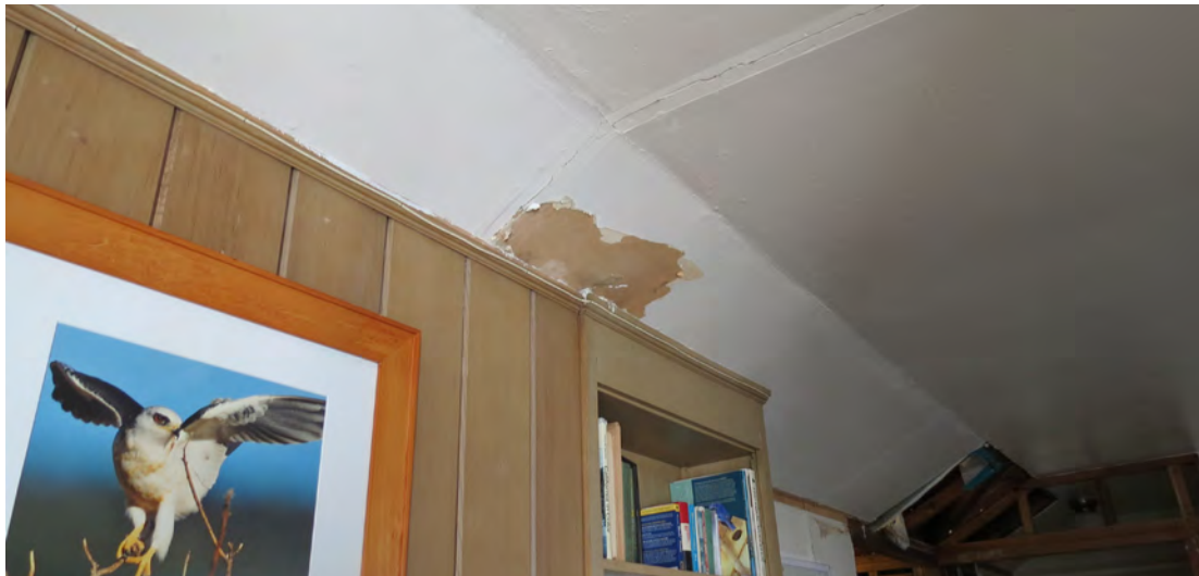
Figure 246. Ceiling damage in Room 103.
