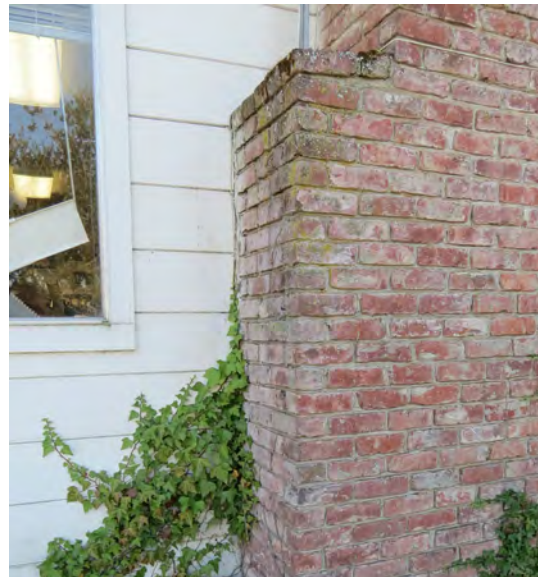
Figure 215. Biological growth on brick chimney at 1960s addition.
