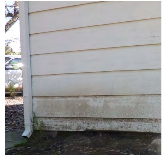
Figure 280. Deterioration and biological growth at siding.
