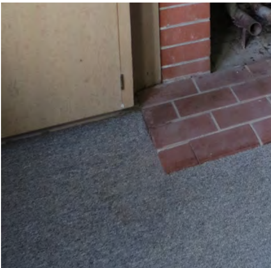
Figure 238. Non-contributing carpet over original Douglas Fir floors in Room 103.
