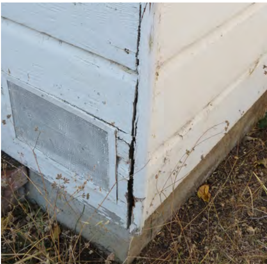
Figure 220. Deteriorating wood siding near foundation.
