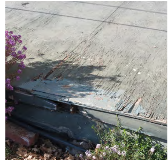
Figure 81. Deteriorating edge of porch.
