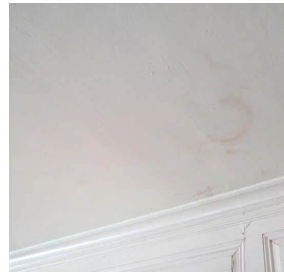
Figure 105. Water damaged gypsum board ceiling in Room 102.
