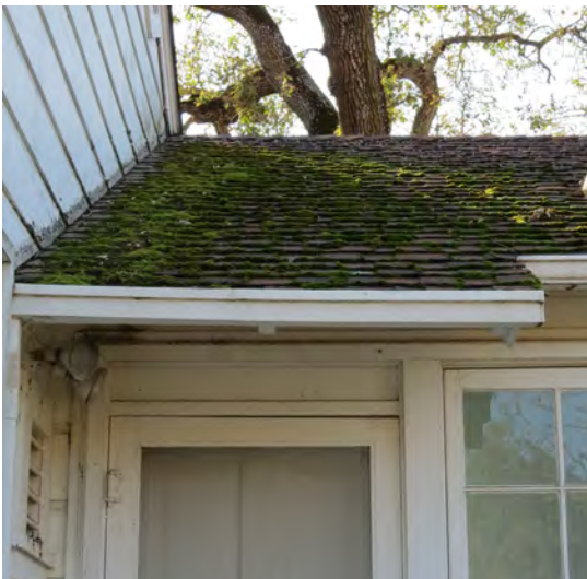
Figure 158. Roof with heavy biological growth.
