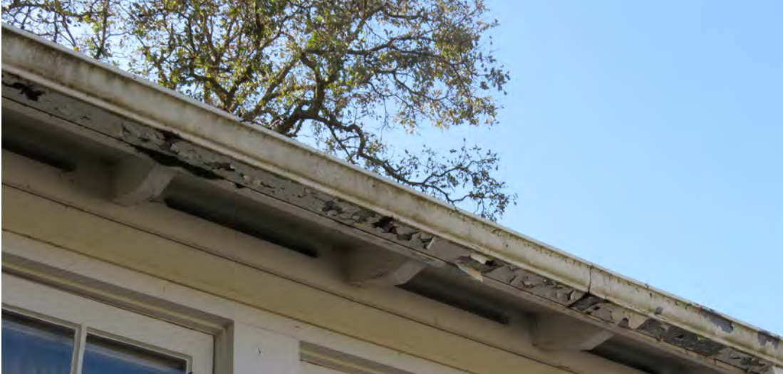
Figure 162. Gutter with severe paint loss on the underside.
