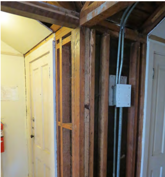
Figure 241. Severe damage at junction between rooms 103, 103A and 103B.
