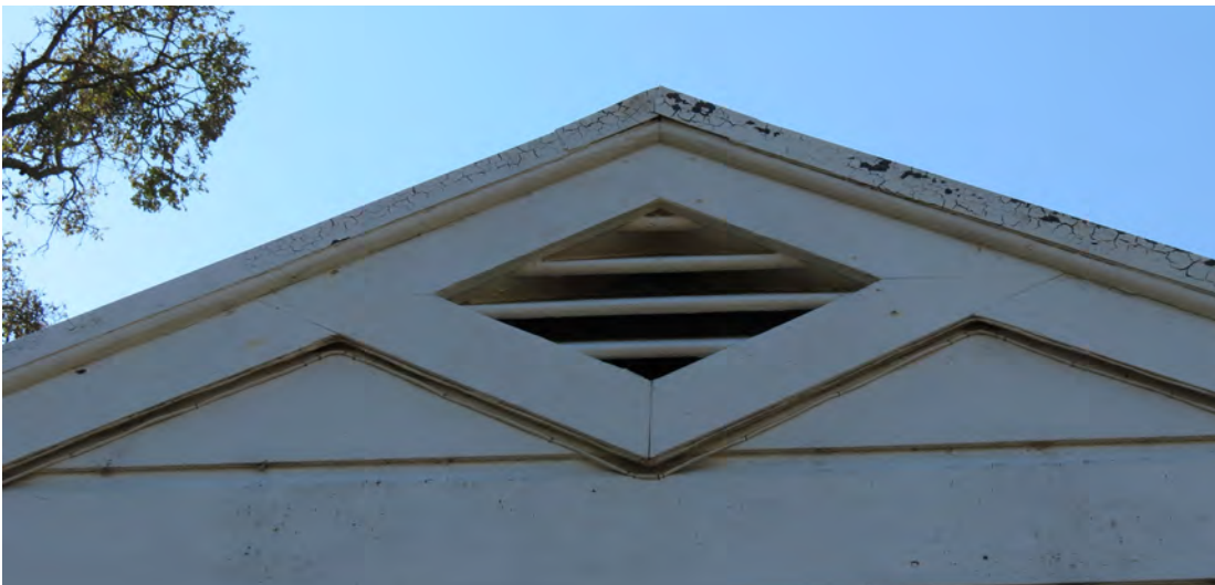
Figure 213. Attic vent and roof flashing with peeling paint.
