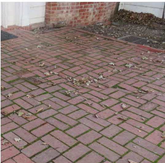
Figure 88. Uneven bricks at entry.
