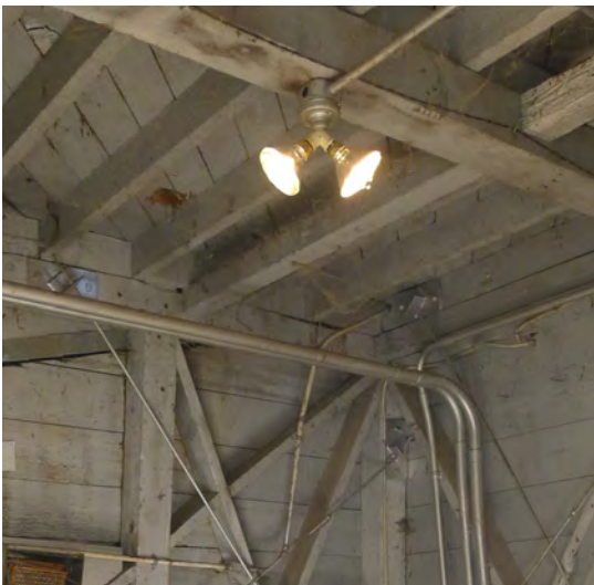
Figure 143. Non-contributing flood light and exposed wood frame ceiling.
