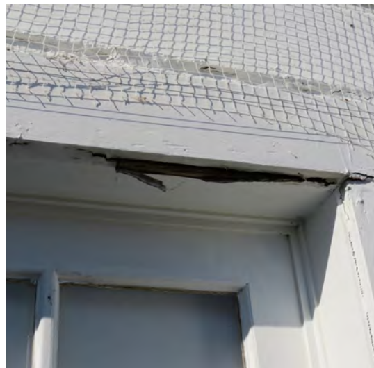
Figure 78. Damaged wood window trim.
