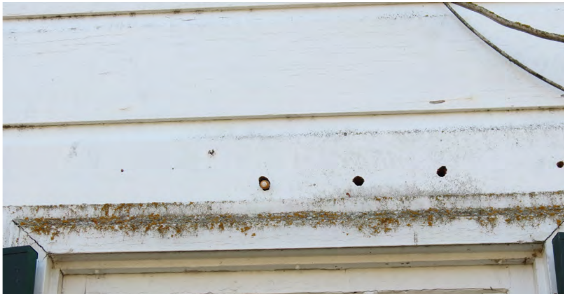
Figure 163. Woodpecker damage to wood siding.
