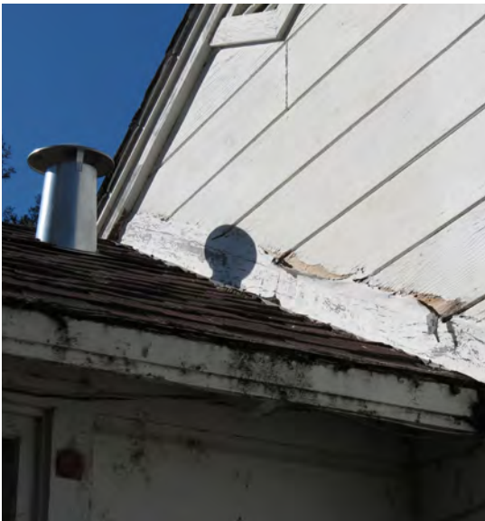
Figure 214. Paint loss at intersection of roof and wood siding.
