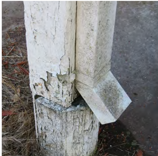
Figure 289. Deterioration at base of posts.
