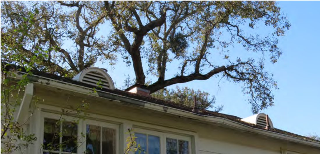
Figure 161. Detached gutter with paint loss.
