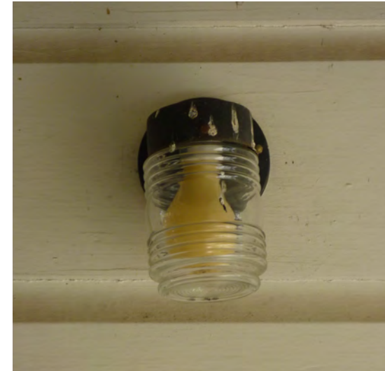
Figure 232. Wall-mounted light fixture.
