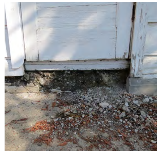
Figure 287. Door and trim deterioration near soil.
