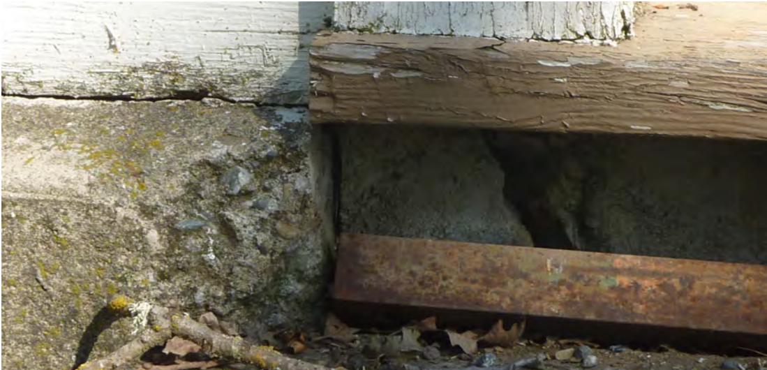
Figure 231. Deteriorating concrete foundation at entry to Room 105 - Wood shed.
