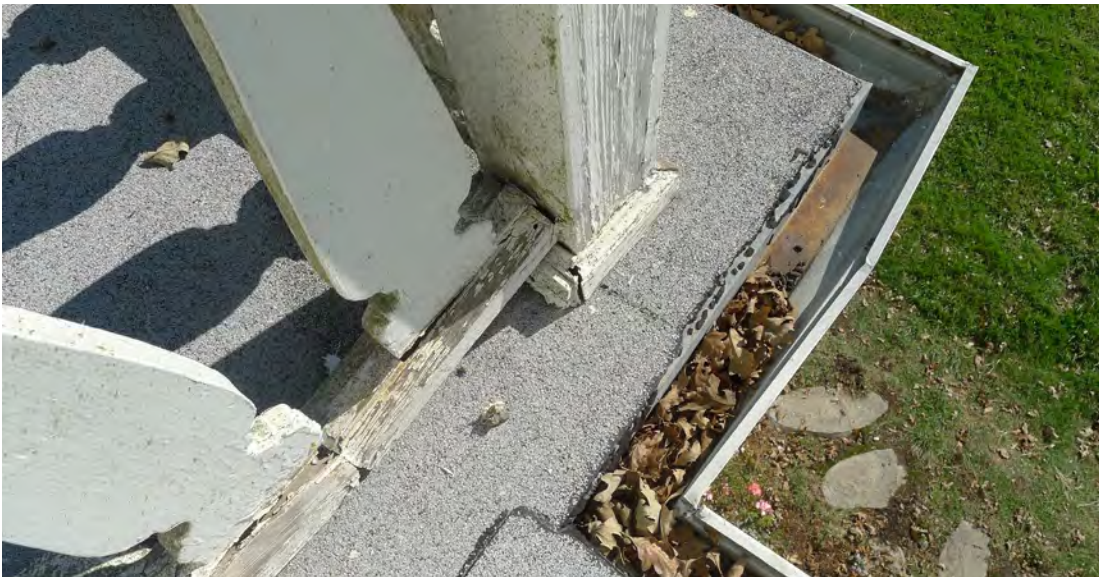
Figure 68. Gutter filled with debris.
