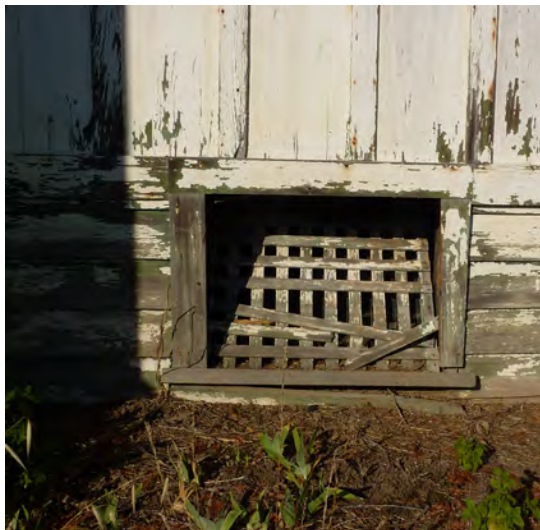
Figure 328. Deteriorated siding and broken foundation vent grille.
