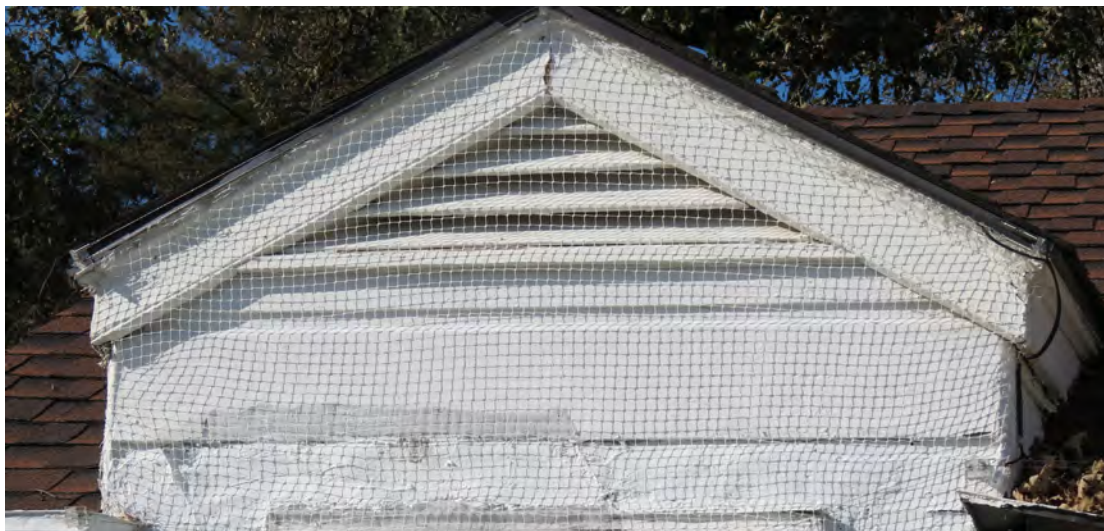
Figure 92. Dormer gable with woodpecker netting.
