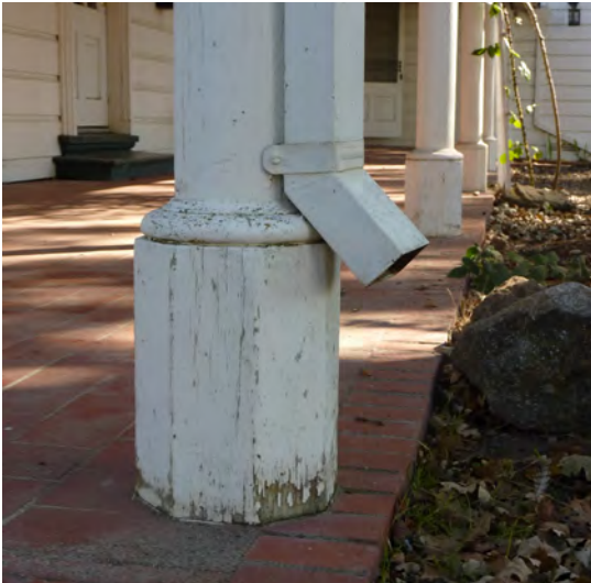
Figure 171. Paint loss at base of column.
