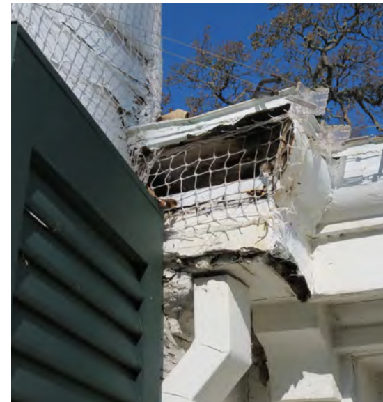
Figure 69. Gutter missing decorative wood molding.
