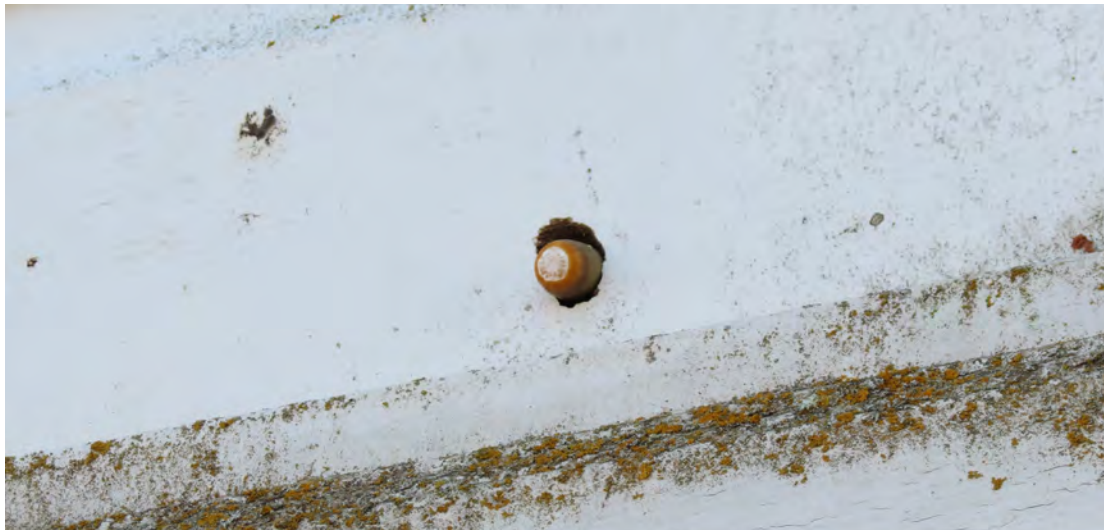
Figure 175. Biological growth and woodpecker damage in siding.
