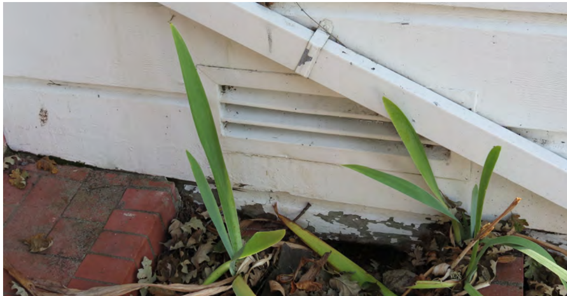
Figure 131. Damaged wood siding in contact with ground.
