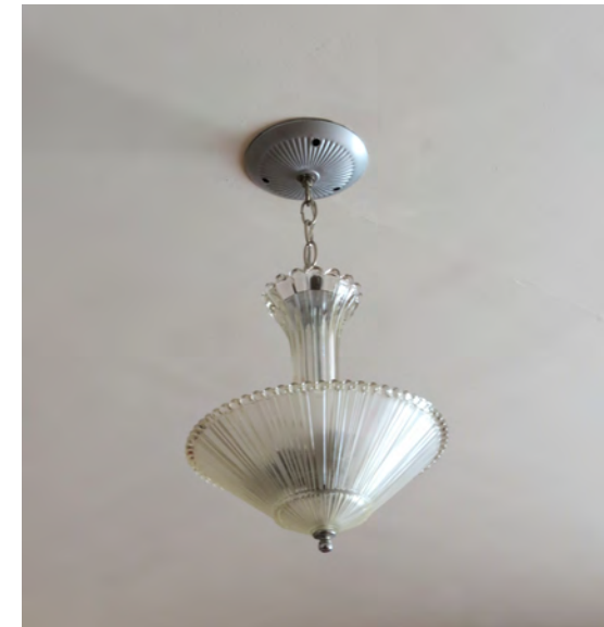
Figure 121. Pendant light fixture with glass shade in Room 109.
