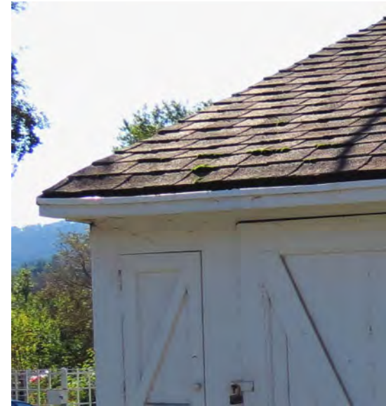
Figure 275. Biological growth on roof shingles.
