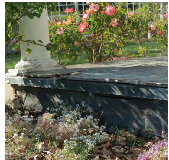
Figure 82. Deteriorating edge of porch.
