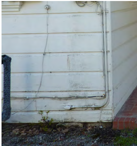
Figure 165. Paint loss and wood deterioration near foundation.
