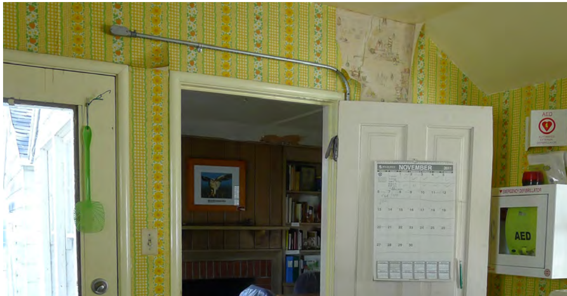
Figure 244. Wallpaper peeling in Room 102 - Kitchen.
