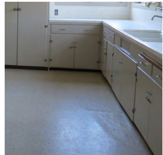
Figure 178. Sheet vinyl flooring in kitchen showing evidence of subfloor damage.
