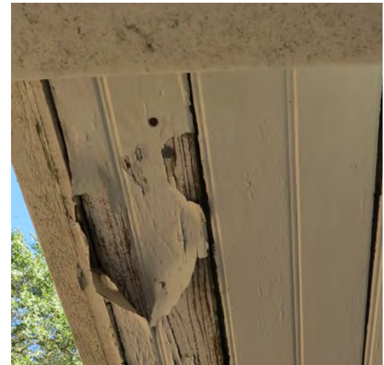
Figure 292. Peeling paint at eaves.
