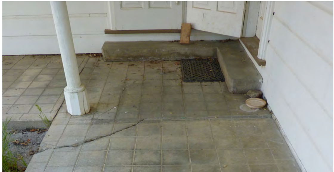
Figure 230. Stamped concrete porch with settlement cracks.
