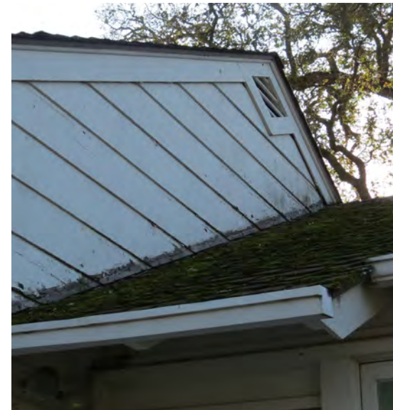
Figure 164. Paint loss and wood deterioration where north addition roof meets siding.
