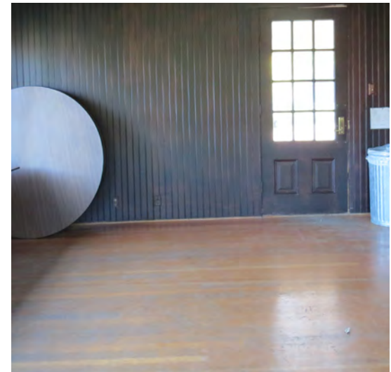
Figure 177. Heavily worn wood floor in Room 101.
