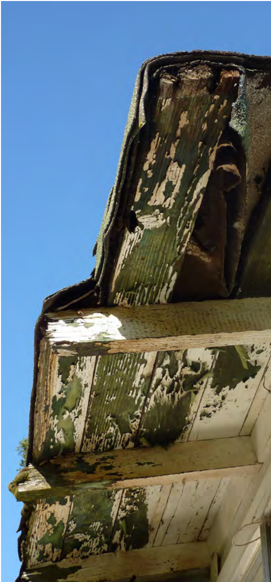
Figure 324. Deteriorated rafters and sheathing.
