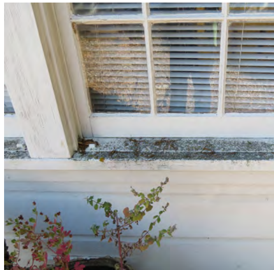
Figure 225. Mold growth on painted wood window sill.
