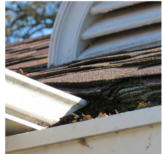
Figure 210. Multiple layers of roofing material.
