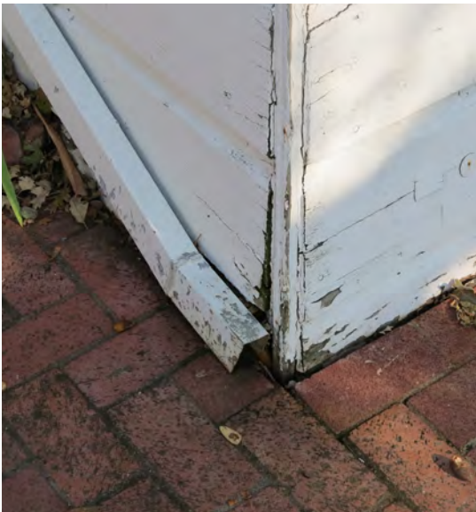
Figure 129. Deteriorating siding at downspout.
