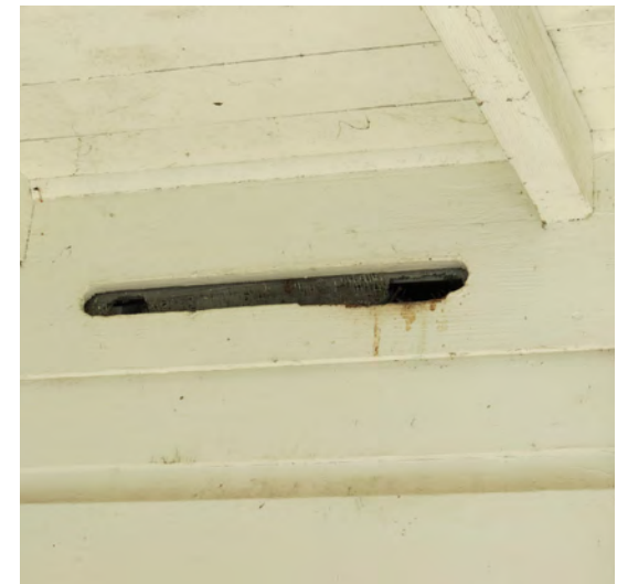
Figure 211. Mesh-covered vent in frieze board.
