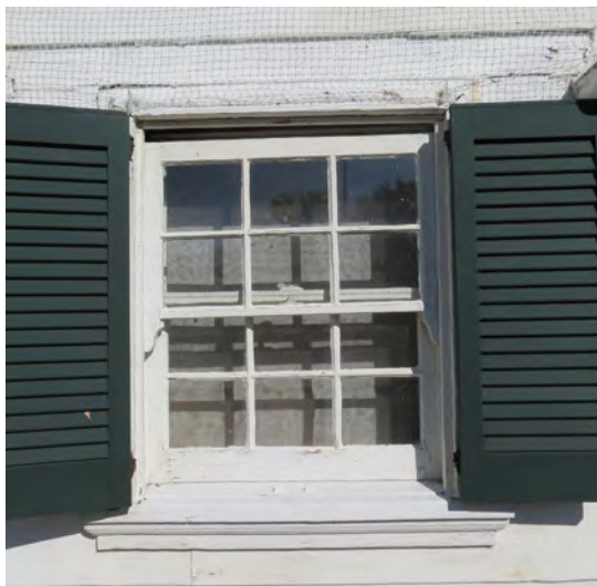
Figure 77. Double hung wood window out of plumb.
