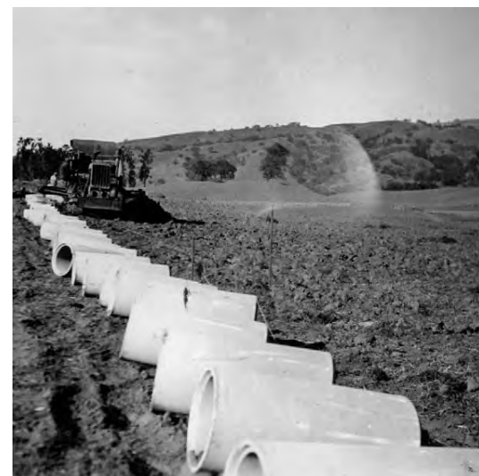
Figure 15. “To Snell,” showing pipeline installation project from lake to Snell agricultural land, 1932. (Grant Park Archives).
