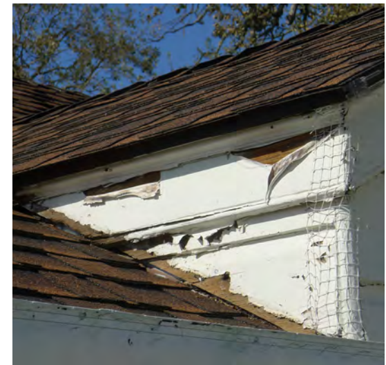
Figure 64. Deteriorating siding on dormers.
