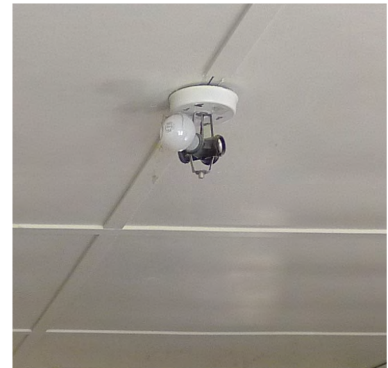
Figure 310. Non-contributing light fixture.
