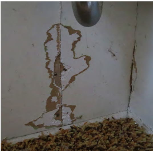
Figure 300. Gypsum board damage.
