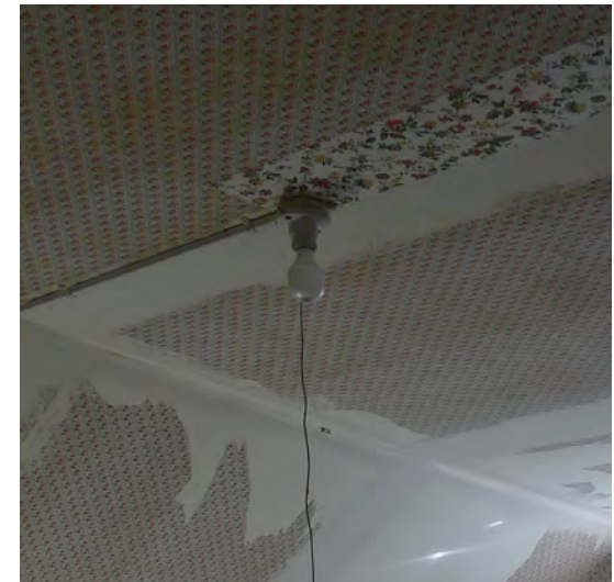
Figure 309. Common ceiling mounted enamel fixture.
