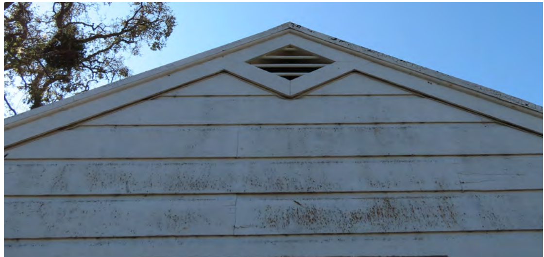
Figure 234. Biological growth staining on wood siding.
