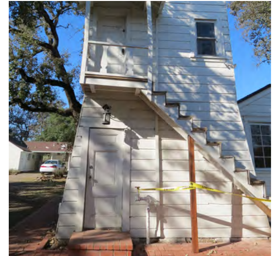
Figure 138. Structurally unstable exterior wood stair.
