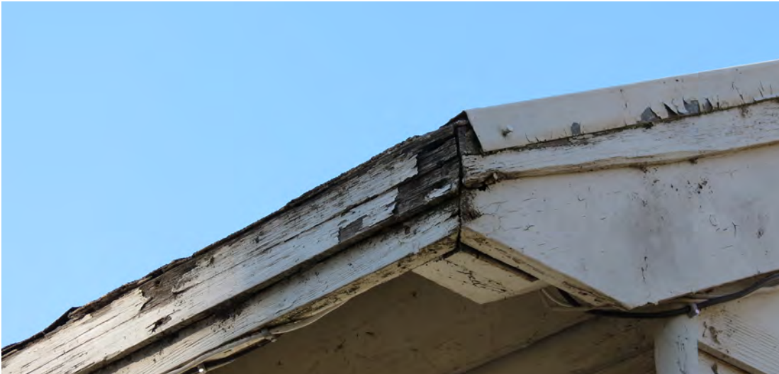
Figure 212. Roof eave with paint loss on wood and flashing and wood deterioration.
