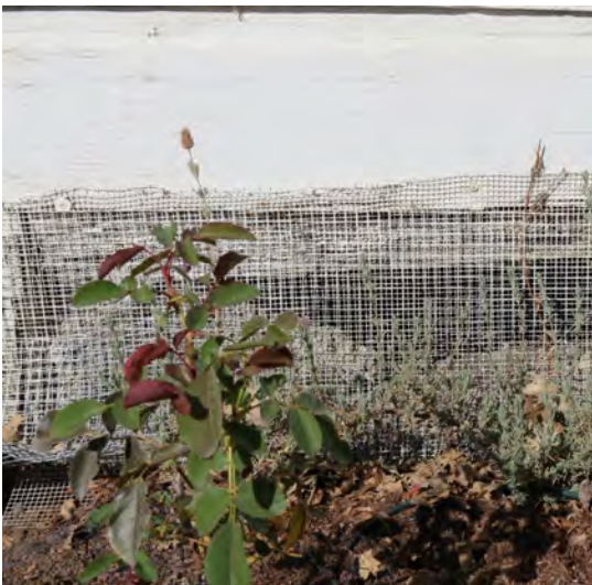
Figure 291. Mesh covering hole at foundation.
