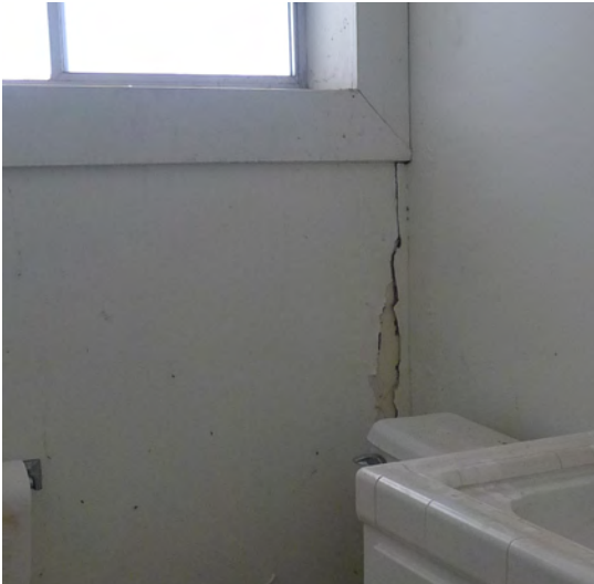
Figure 299. Crack under window in Room 110.
