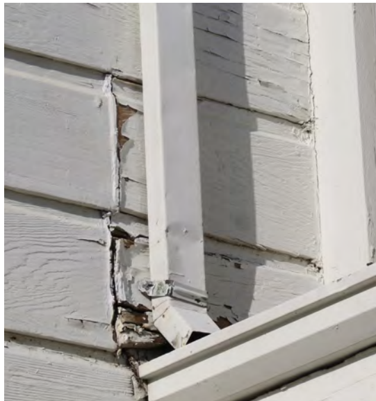
Figure 70. Damaged wood siding at downspout.
