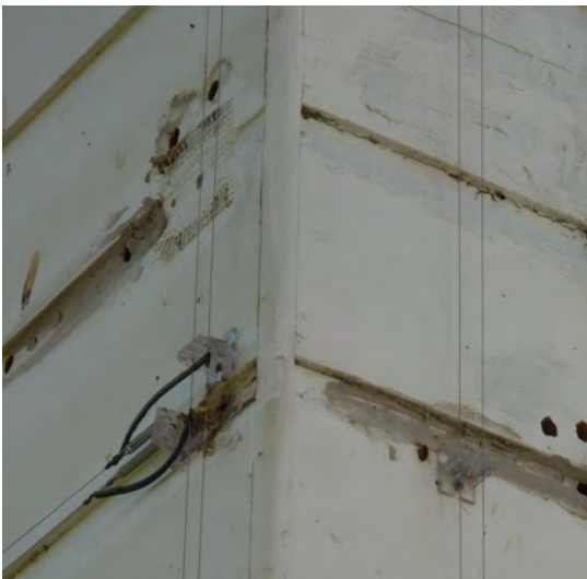
Figure 73. Woodpecker damage to siding.
