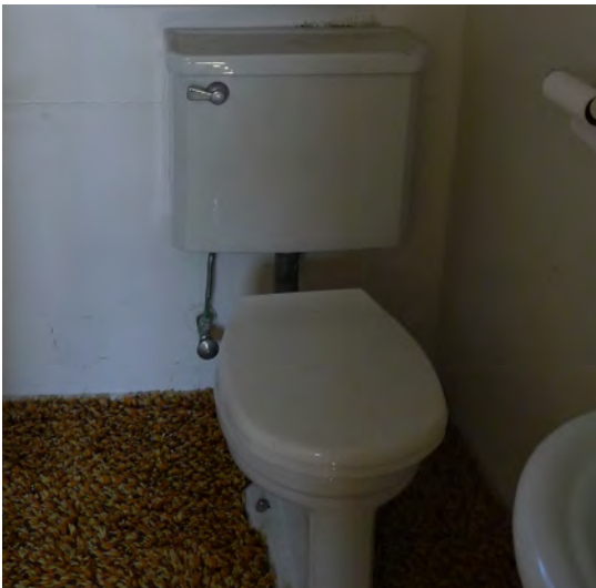
Figure 307. Original plumbing fixture.
