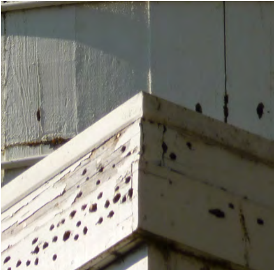
Figure 136. Woodpecker damage and missing paint at fascia.
