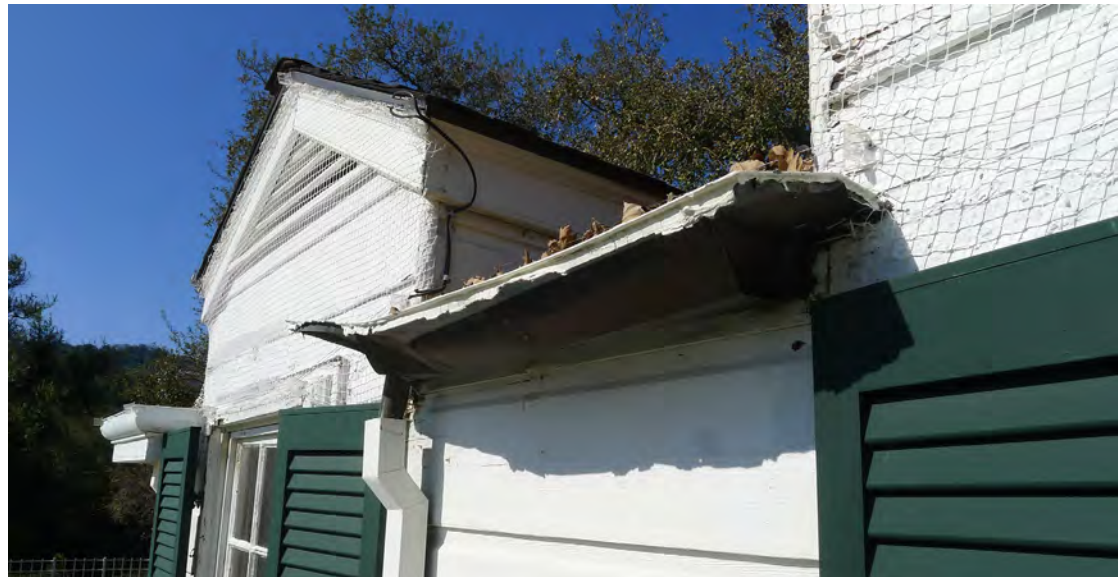
Figure 71. Gutter missing decorative wood molding.
