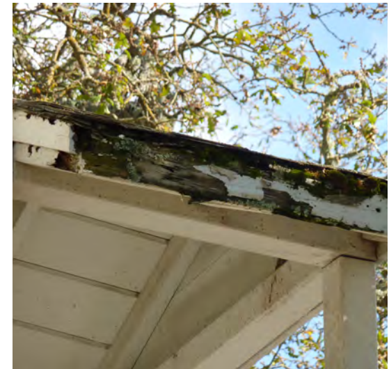
Figure 127. Biological growth at second floor gable roof.
