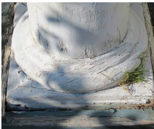
Figure 80. Paint loss at base of wood column.
