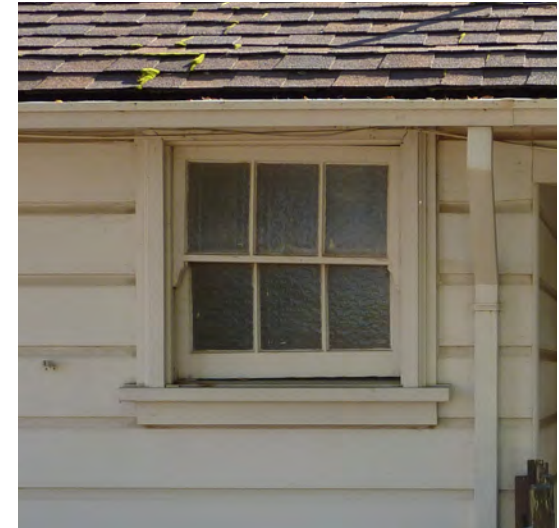
Figure 224. Out-of-plumb double hung wood window.
