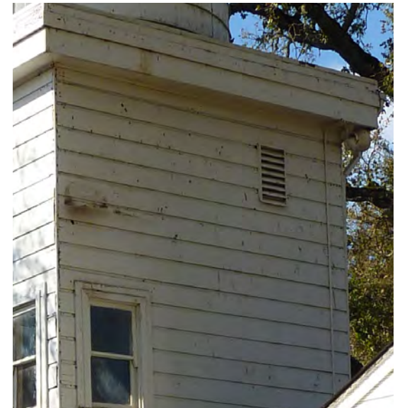
Figure 132. Damaged siding on northeast elevation of Tank House.
