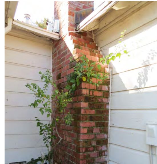
Figure 216. Biological growth and vegetation on chimney at 1937 addition.
