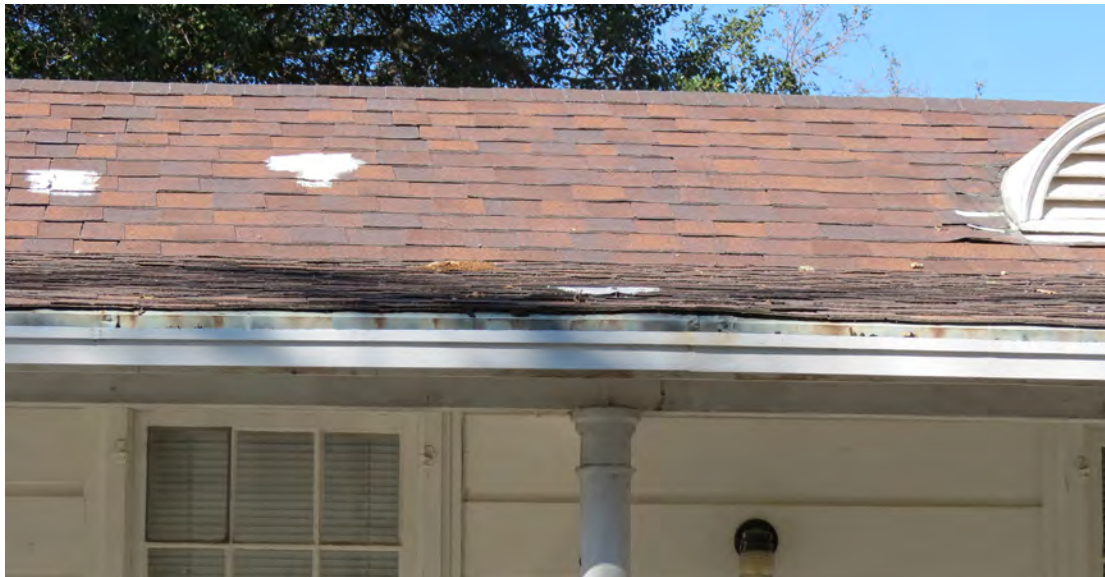
Figure 217. Damaged gutter and rusted flashing.
