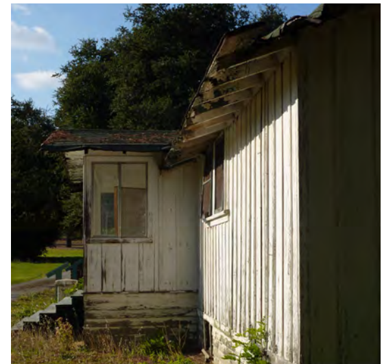
Figure 326. McCreery Cottage with no drainage system.
