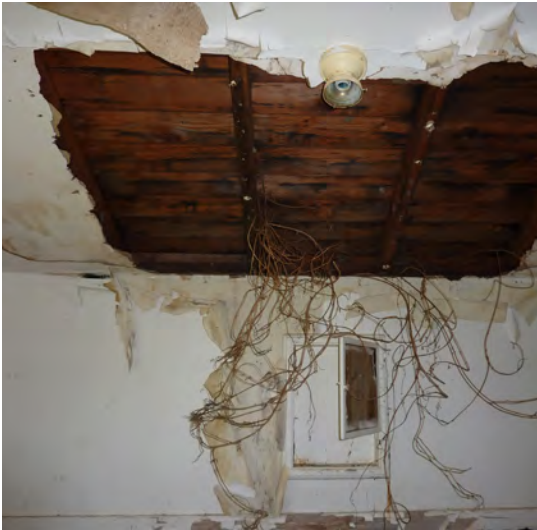
Figure 343. Damaged gypsum board ceiling in Room 105.
