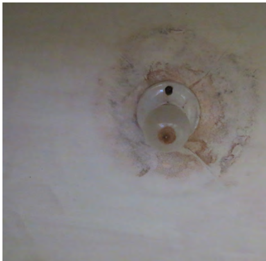
Figure 103. Water damage around light fixture in closet 105B.
