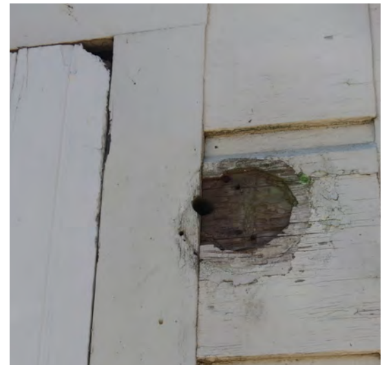
Figure 281. Large hole from removed light fixture.
