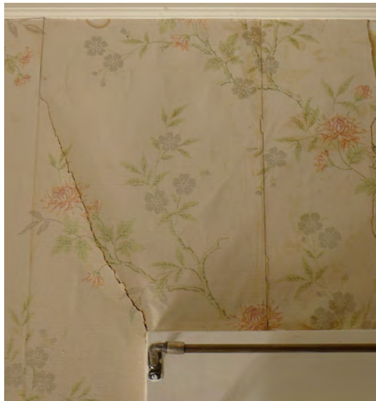
Figure 99. Cracked gypsum board and wallpaper in Room 109.
